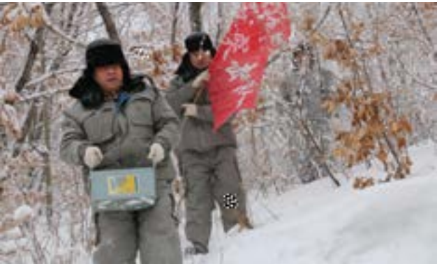
The Longyuan Heilongjiang Company 's Bianfushan Wind Farm fully played the role of the youth power in the 80-day ensuring safety and increasing power generation corporate competition. Young employees rushed over the snow for repairing the wind tower battery feed failure, making every effort to ensure the safe and stable operation of the wind farm.
